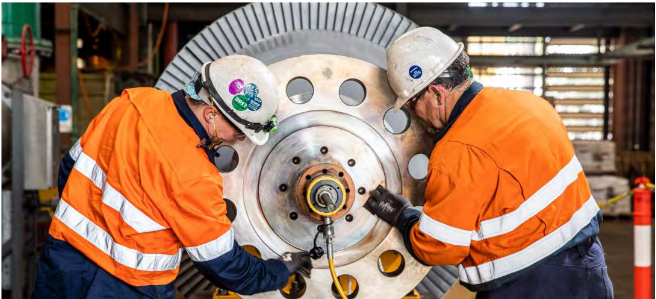
Photo: Overhaul contractors work on the Callide Unit B2 HIP turbine rotor during the unit's overhaul in FY2019.
